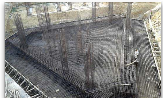
VYOM used STAAD to arrange the columns so that the lateral force will rest completely on the center of the building.
