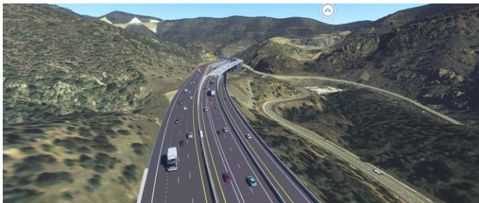
The Floyd Hill roadway upgrade will improve safety and mobility along a congested eight-mile stretch of Colorado’s I-70 mountain corridor.
